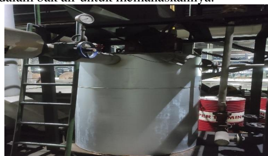
Gambar 1. Thermal oil heater
