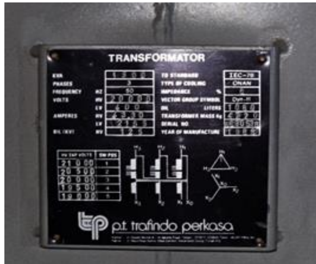
Gambar 7. Name Plate Transformator
